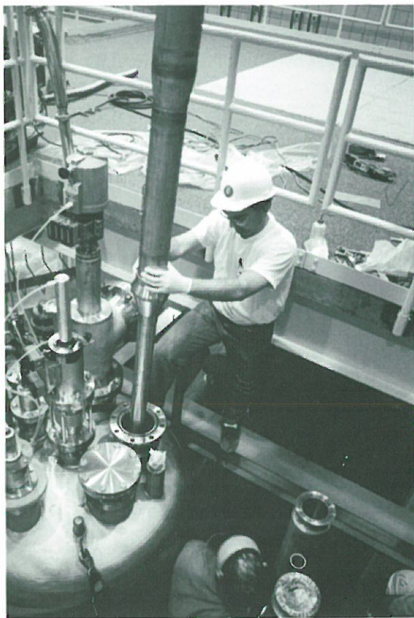
Test of the 10kA current leads of the hybrid magnet.
