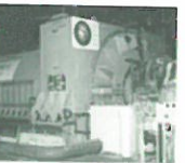
6. The 1.43 GVA motor-generator at Los Alamos. The generator will be used to power the 60 T quasi-continuous and non-destructive 100 T magnets.
