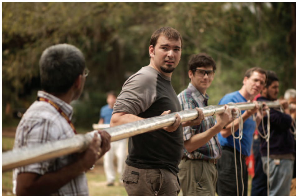
ABOVE: From administrators to students to facilities personnel, all hands were on deck for the installation of long sections of underground pipe as part of the lab's ongoing effort to improve helium recovery & economy. The project has already resulted in dramatically reduced helium usage. (Photo by Dave Barfield)
