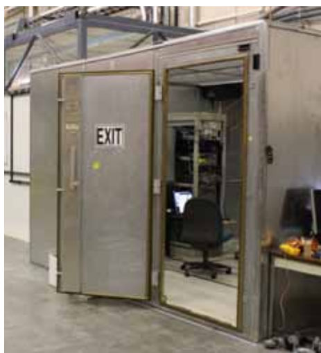
FIGURE 1. A new electromagnetically screened room (shown above) and heavy wall copper conduit was installed.
