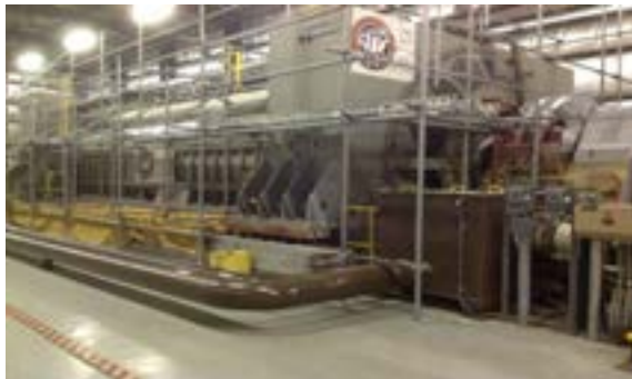
Figure 8: The 1.4 billion watt generator gets a careful inspection and review before a fresh coat of paint in 2014. LANL paid for the entire operation.
