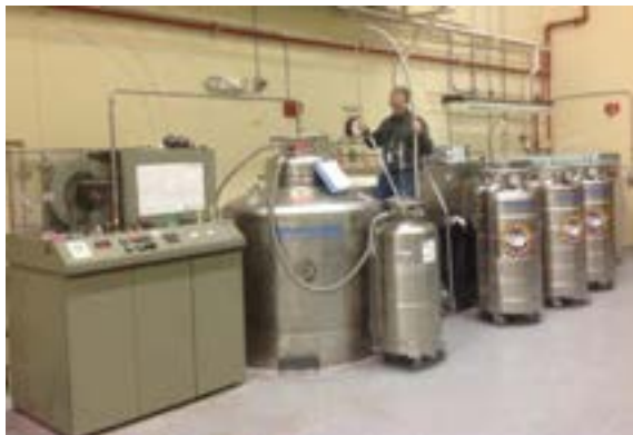
Figure 4: The now operational liquid helium recovery and liquefaction system at the NHMFL-PFF.
