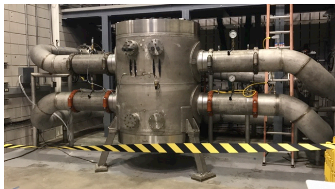
Figure 5: 41T resistive magnet located in cell 6.
