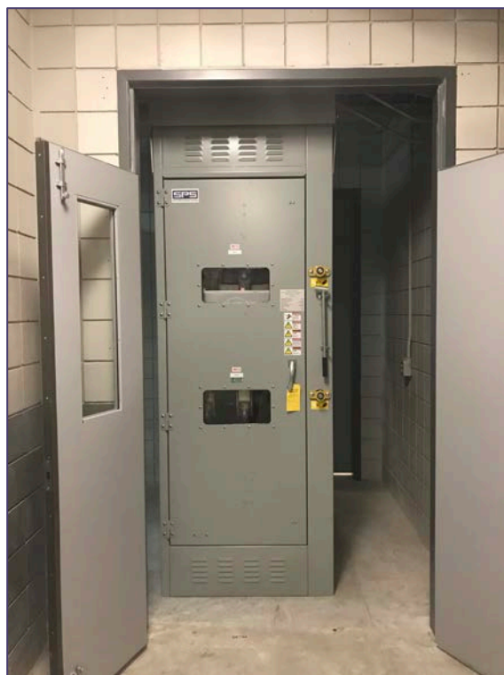
Figure 2.b.2: 12.5 kV Power supply disconnect for power supply A and B.
