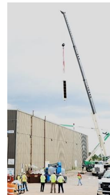
Figure 2.2.7.2.2: The cleaning of the 4 motor generator coolers required removing each 16-foot tall and 7,500lbs. cooling towers via a small hatch in the roof above each corner of the motor generator. The teams responsible for this high consequence operation included LANL, PFF, and external contactor personnel.
