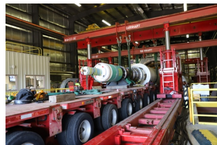
Figure 2.2.7.1: The removal of the 1.4GW motor-generator rotor in preparation for a full inspection at GE in Richmond, VA.
