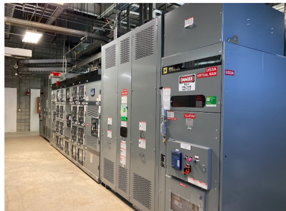
Figure 2.2.2.2: Three-phase 12.5kV-480V switchgear
