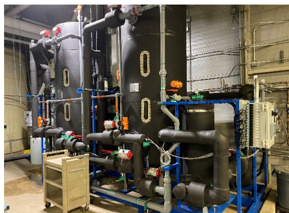
Figure 2.2.2.1: New magnet cooling water treatment system
