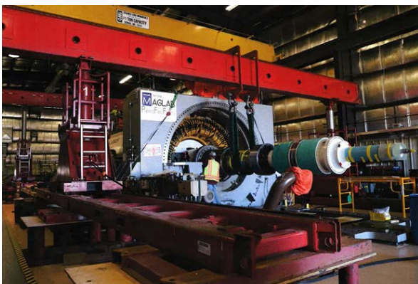
Figure 4.4.13: The rotor was removed from generator housing for further investigation and repair (September 2019).
